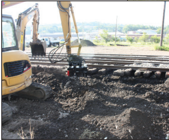
Photo at left shows BB10.4G at work on Caterpillar 314 excavator, with Cat 305 working along side digging the trench for the fouled ballast.
